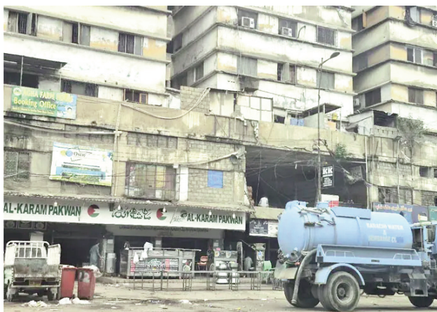
Dilapidated buildings on a littered road in Karachi's FB Area: across the city, residential and commercial façades stand unwashed and unpainted, sometimes for decades | Photos by the writer
