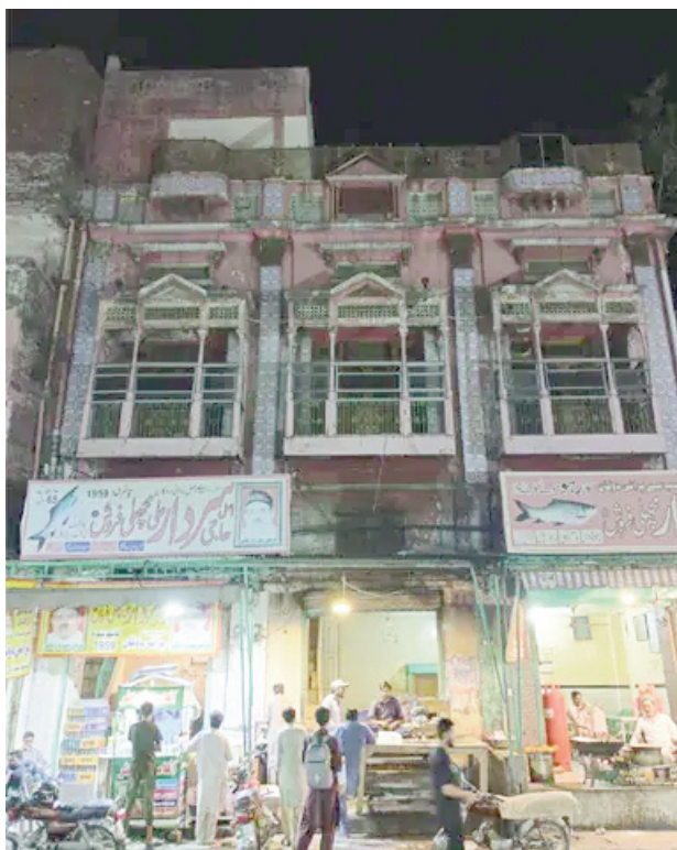
A handful of customers at a famous fish shop in Gawalmandi, with the beautiful façade of the structure above it in need of restoration | Photo by the writer
